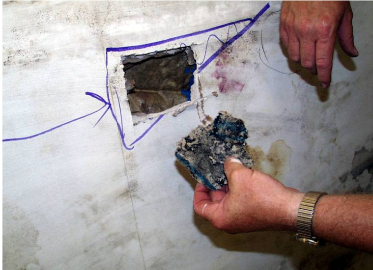
Figure 2. Mold found inside a wall by finding moisture indications with IR.
