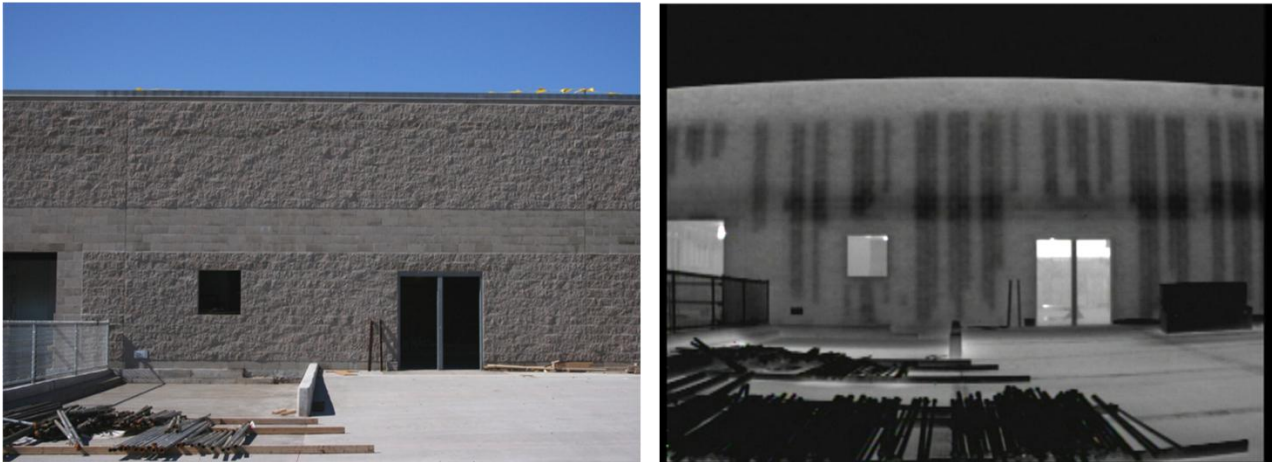
Figures 3. Visual and IR image of CMU building wall. (Grouted areas are lighter.)
