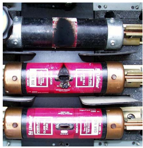
Figure 6 – Fused disconnect showing blown fuse.
