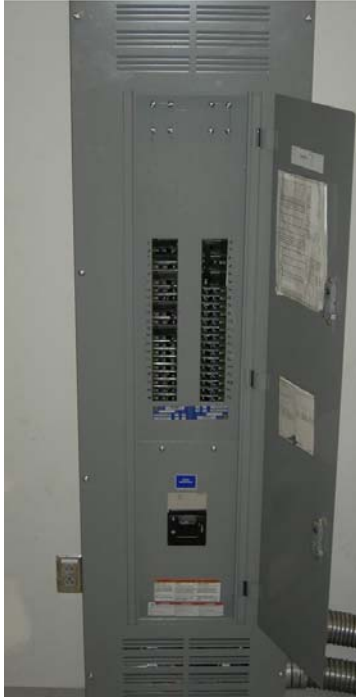
Figure 1 – Typical electrical panel
