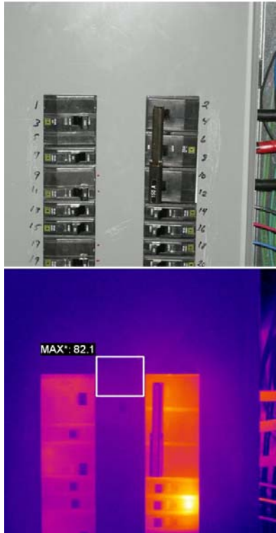
Figure 3 – Visual and thermal image of a panel with only the deadfront cover on.
