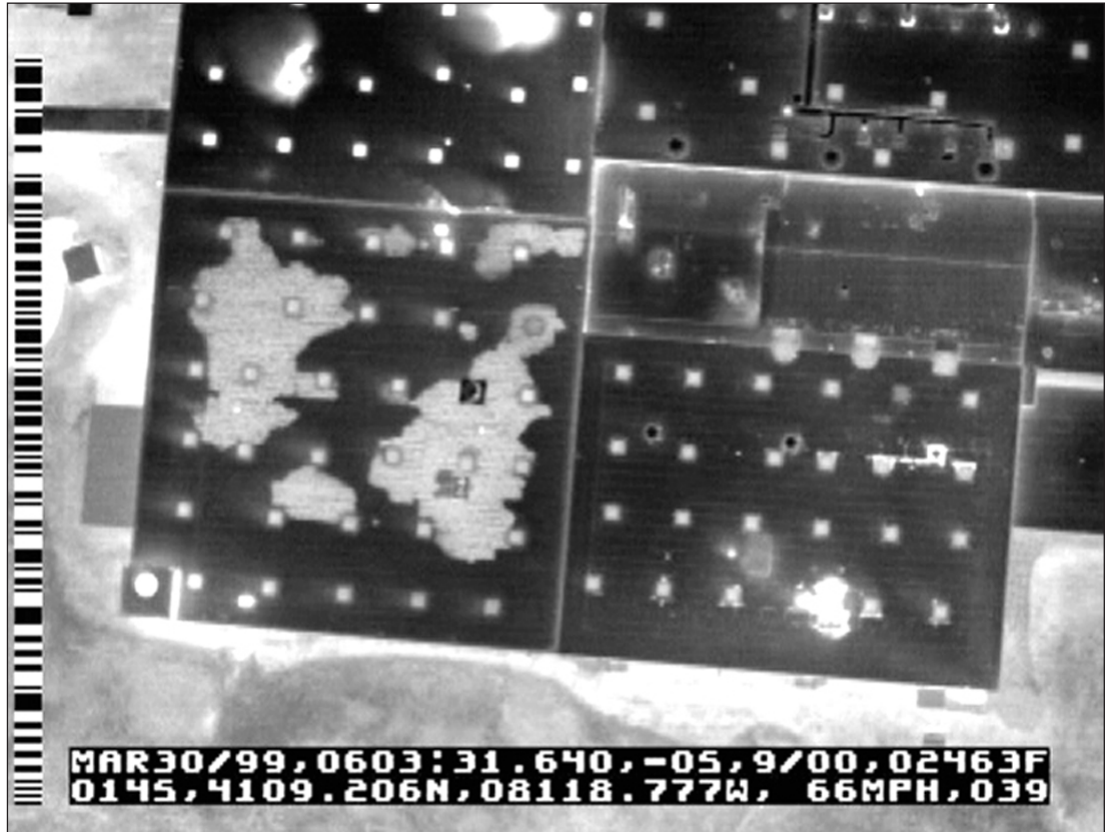
Figure 1: Aerial infrared thermograph taken from 2000 ft. over the building, showing crystal clear outlines of subsurface roof moisture. Light colored areas contain moisture. Dark areas are dry.
